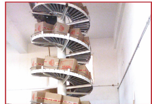
Spiral Conveyor from Top Floor to Ground CB Transfer
